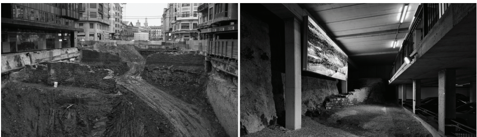
Figure 18. Incorporation of archaeological remains into the underground car park in the Carlos III Ave.
