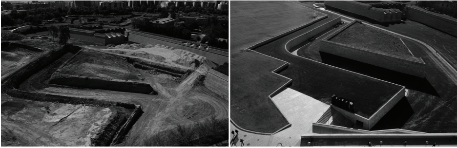
Figure 16. Santa Lucía Ravelin: state during and at the final stage of the excavation.
