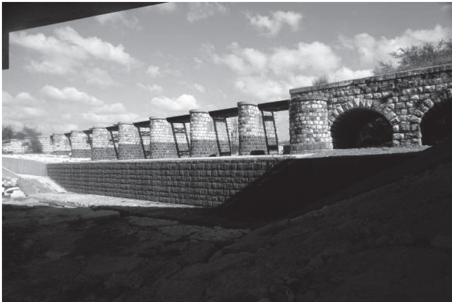
Figure 1. Te'enimRiver Bridge. Restored by Trans-Israel highways management corporation Ltd as part of highway 6 development project. Executed 1999-2008.
