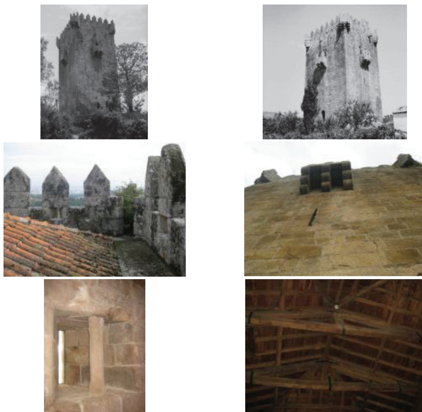
Figure 1. Various views from the Quintela tower: (a) northwest and northeast facades, (b) southwest and southeast facades, (c) views of the roof and border surrounded by battlement with merlons, (d) slit and balconies, (e) slit openings from the interior and (f) view of the trusses and roof.
