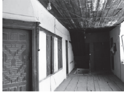
Figure 40. Case03 Situation of external sofa space, deterioration of the wooden material of sofa ceiling.
