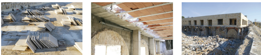
Figure 10. Manual removal of the terrace stone tiles (left), disconnecting the structure of the restaurant from the perimeter of the wall (center) and demolition of restaurant structures (right).
