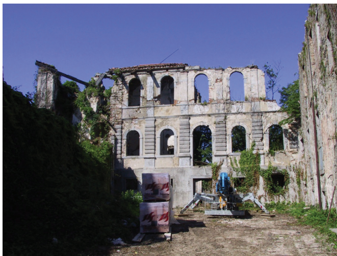
Figure 16. The west front of the East wing after the earthquake.
