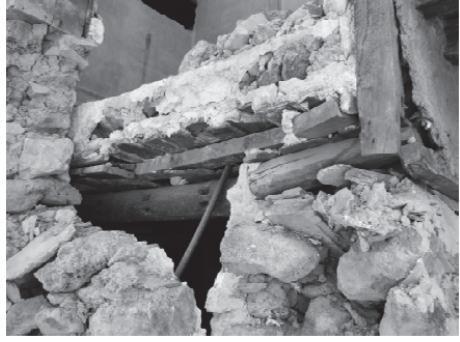
Figure 62. Case09 The deteriorated timber elements and masonry wall.
