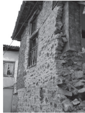
Figure 64. Case09 The collapsed part of the house.
