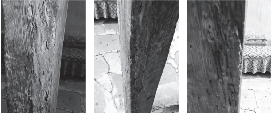
Figures 44, 45 & 46. Case04 Deterioration Problems of the Posts (Color change, holes caused by insects and sectional material loss).
