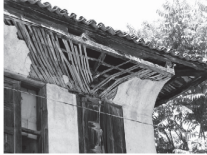
Figure 56. Case07 Material Loss on the Eaves of the building.
