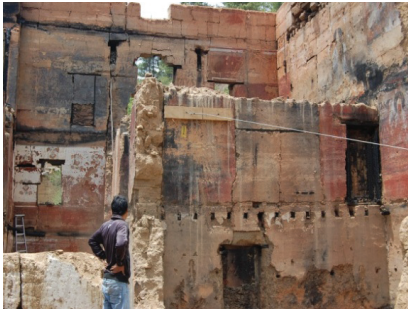
(a) Wall-1 (out-of-plane).
