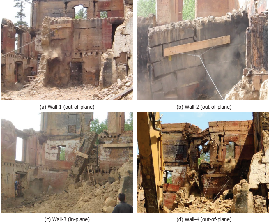
Figure 12. Collapse mode of rammed earth walls.
