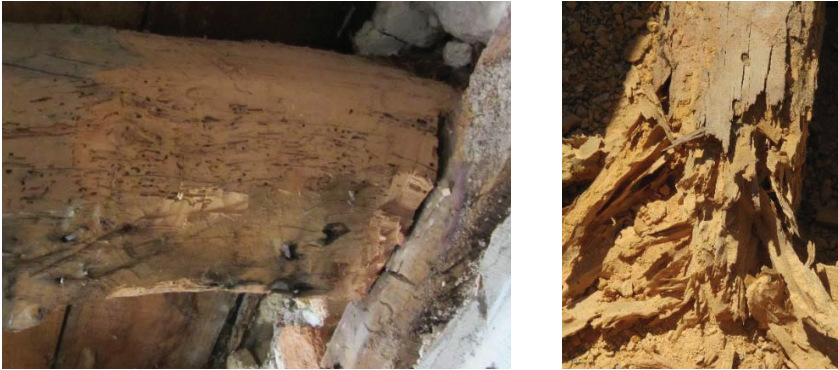
Figure 1. Examples of decayed old timber end beams.
