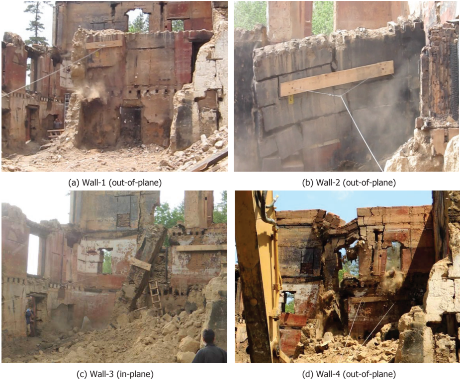
Figure 12. Collapse mode of rammed earth walls.
